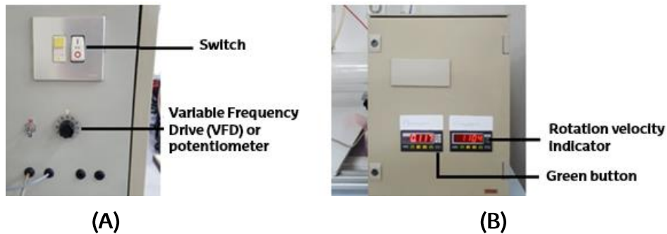
Figure 2: A: Switch to turn on fan and frequency controller or potentiometer. B: Power display and rotation speed.
