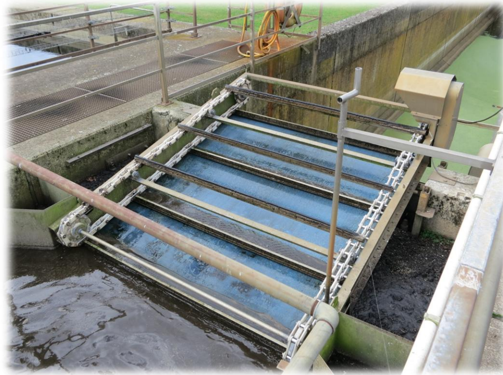
Screens used in a wastewater plant
