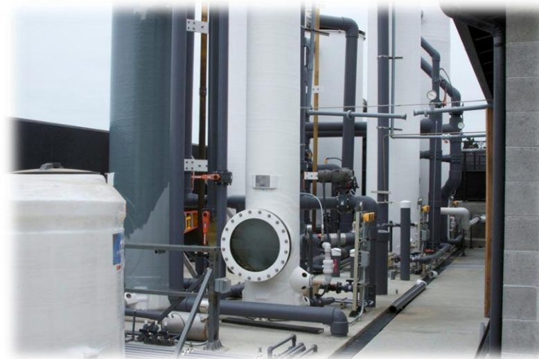
Ozone disinfection system
