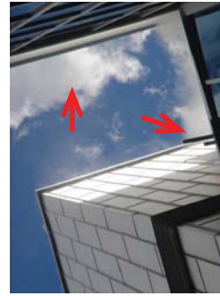
Figure 19: Excessive smoke exfiltration was clearly visible at the top portion of the CW assembly.
