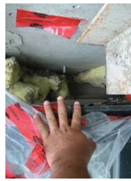
Figure 29: Close-up view of figure 28 - no air seal at the interface detail (the polyethylene sheet was installed as a temporary measure after removing the masonry).
