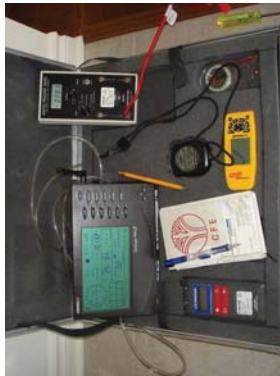
Figure 11: Monitoring panel equipped with remote weather station receiver and digital micro manometers.
