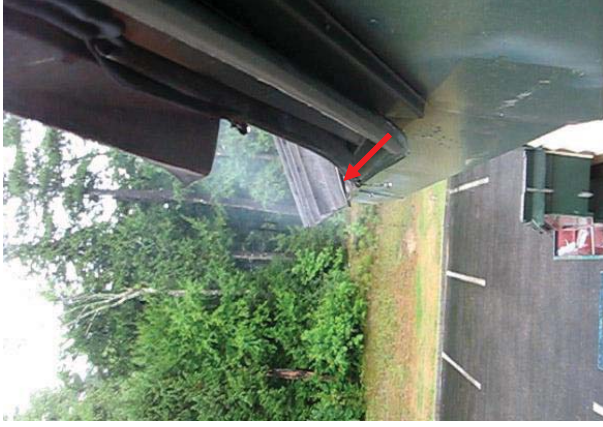
Photo 3: Tracer smoke exfiltration at roof eave (arrow).
