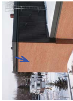
Figure 23: Thermogram of bottom CW section with building under negative pressure.
